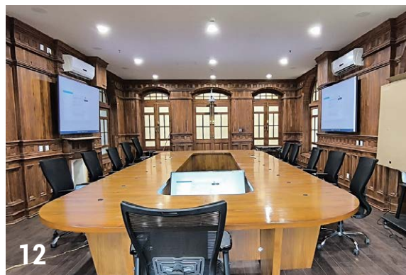
Pink Noise Professionals and Omsan Smart Technologies install state-of-the-art audio equipment at Audit Office, Shimla
